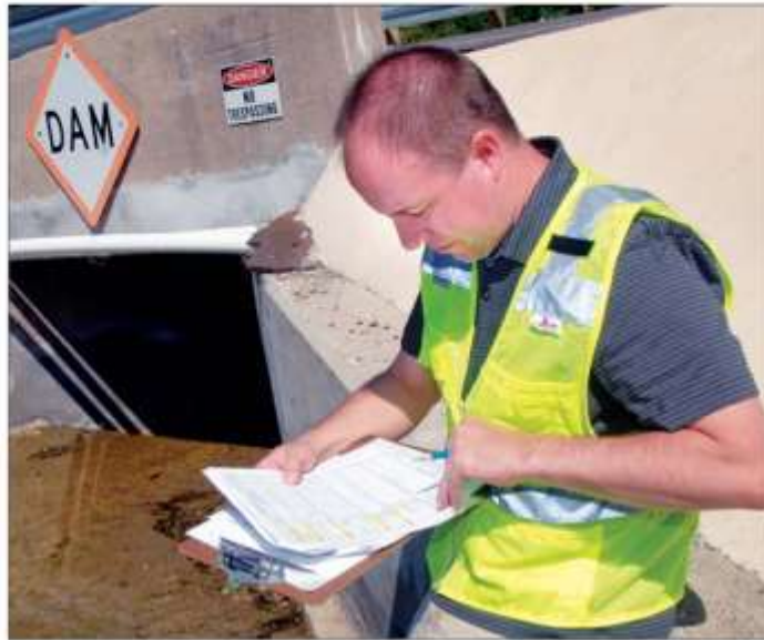
Paul Wirth of Patrick Engineering looks over records and makes notes during an inspection of the Lake Beulah dam area late last month. The earthen dam is No. 5 on a priority list of 15 publicly owned dams across the state that need to be repaired, abandoned or removed.
